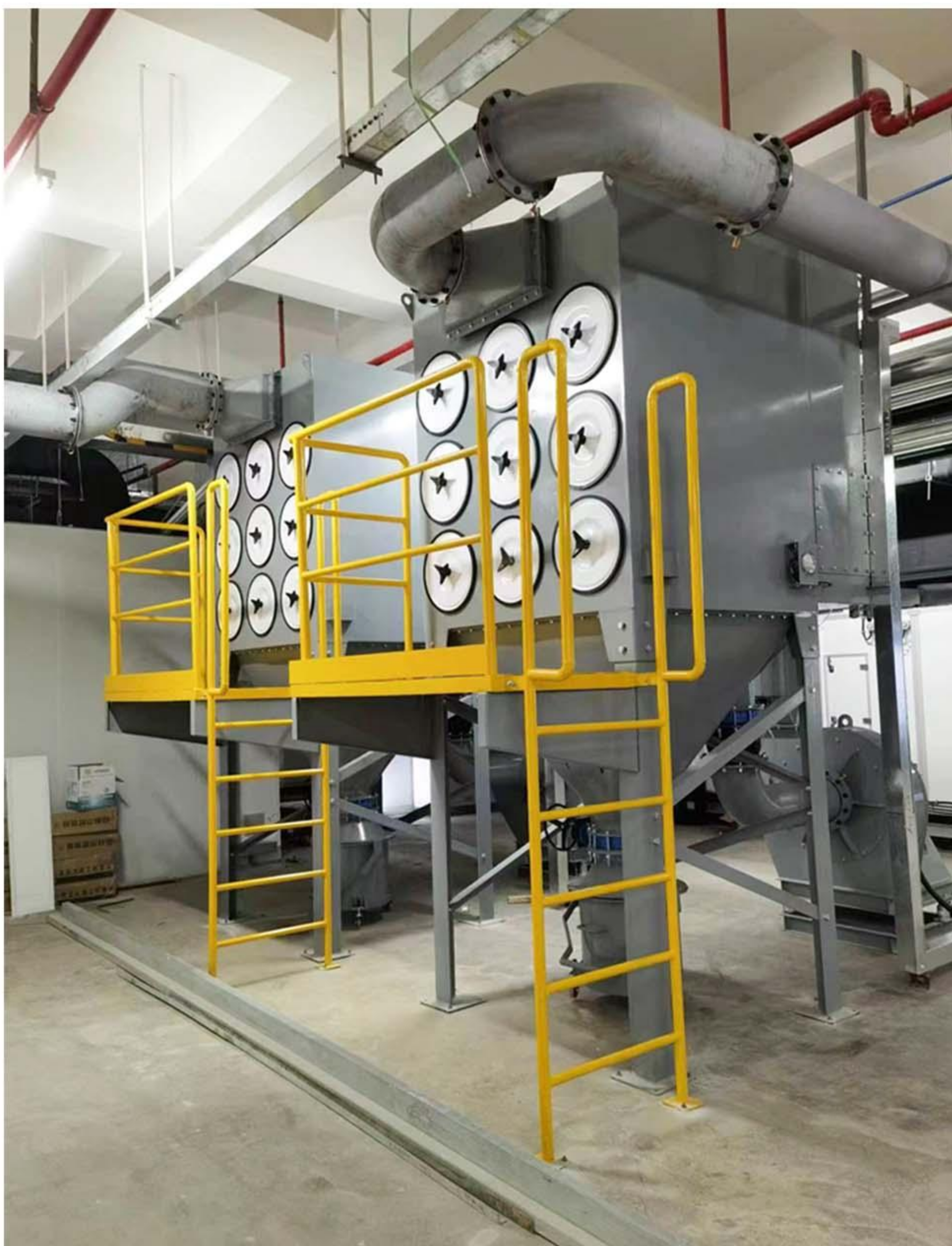
CCL (Copper Clad Laminate) Industry Dust Collection System - Hangzhou
