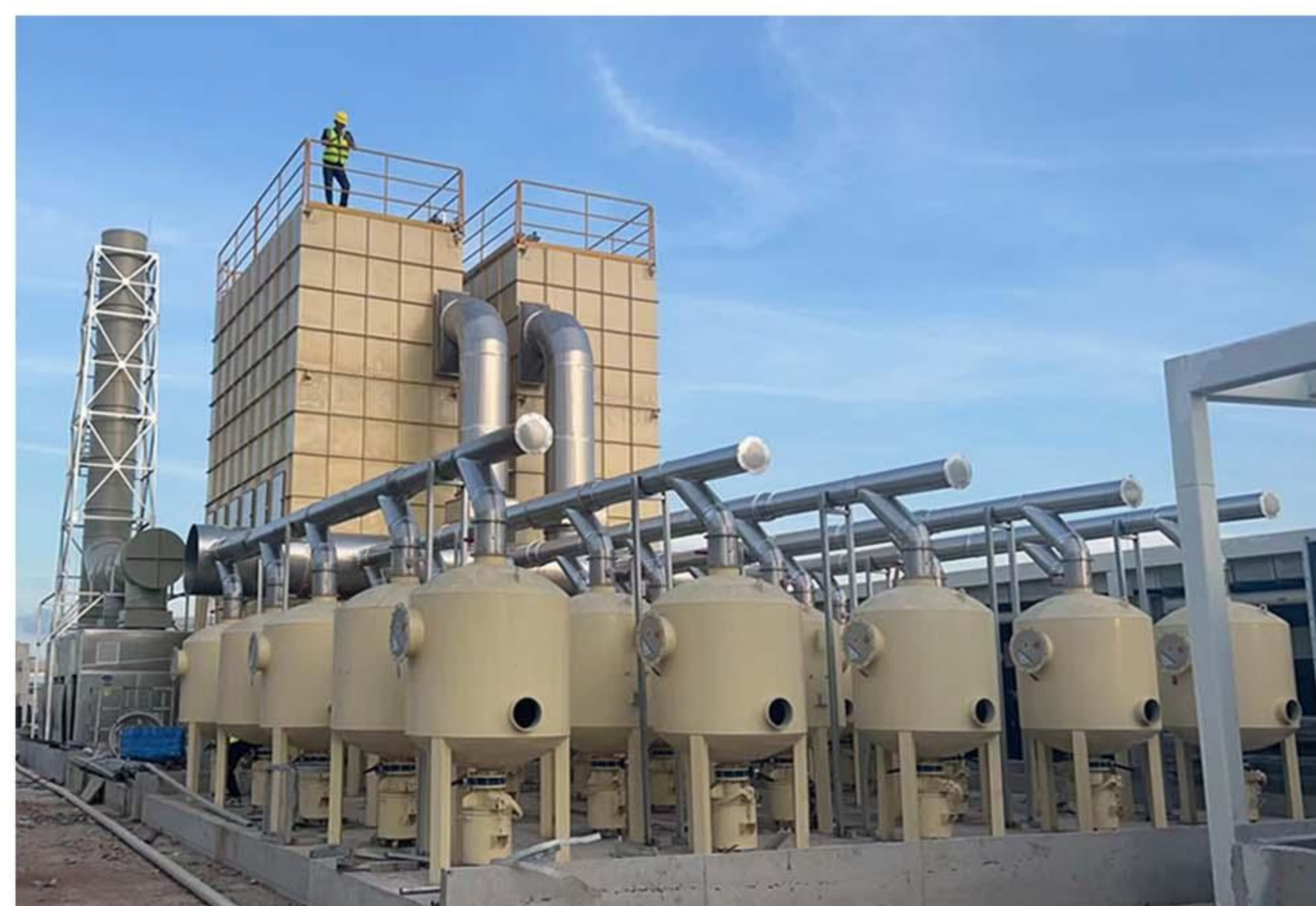
Dust Collection System for Photovoltaic Module Factory - Ningbo
