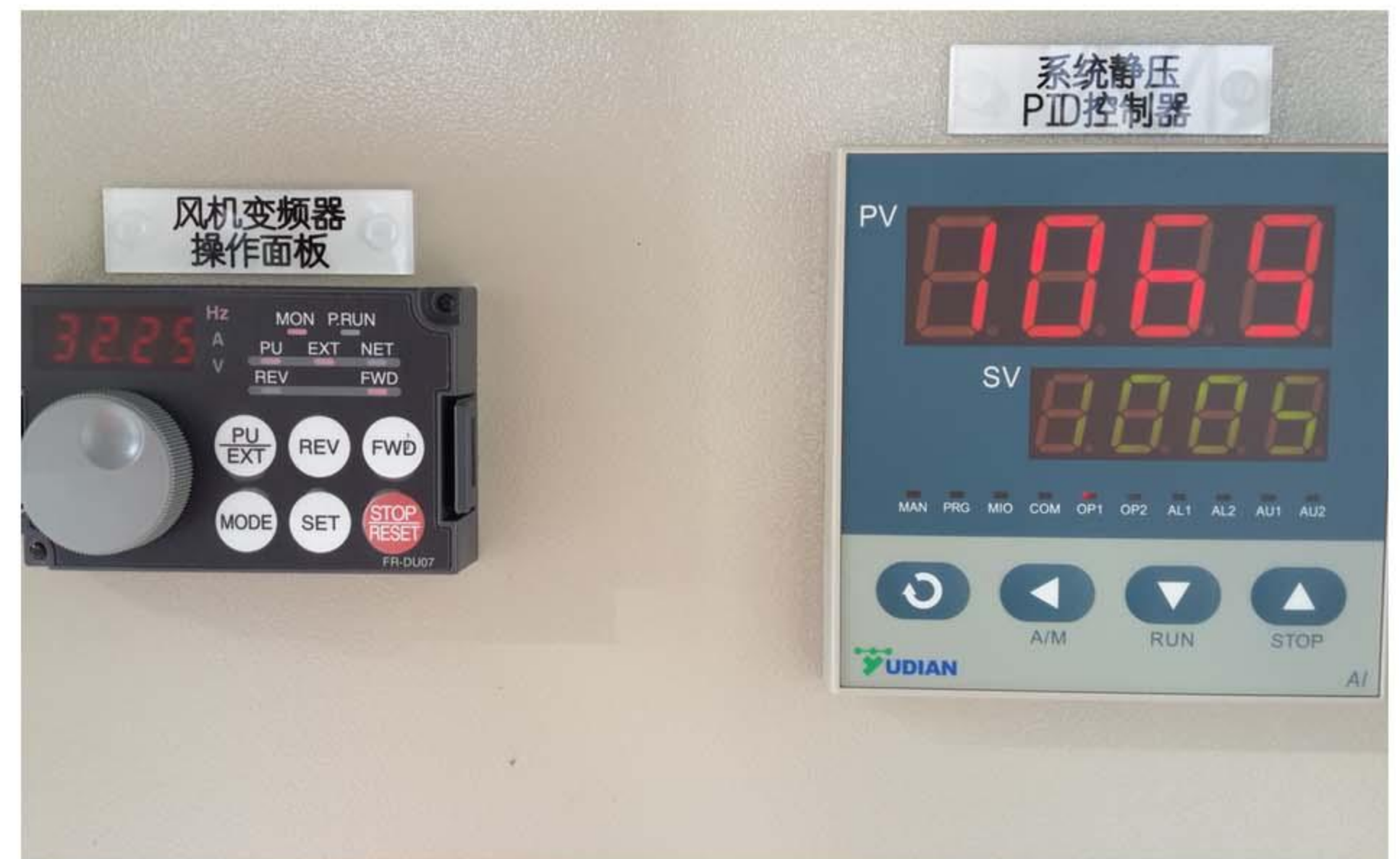
Control System of Scrubber Tower
