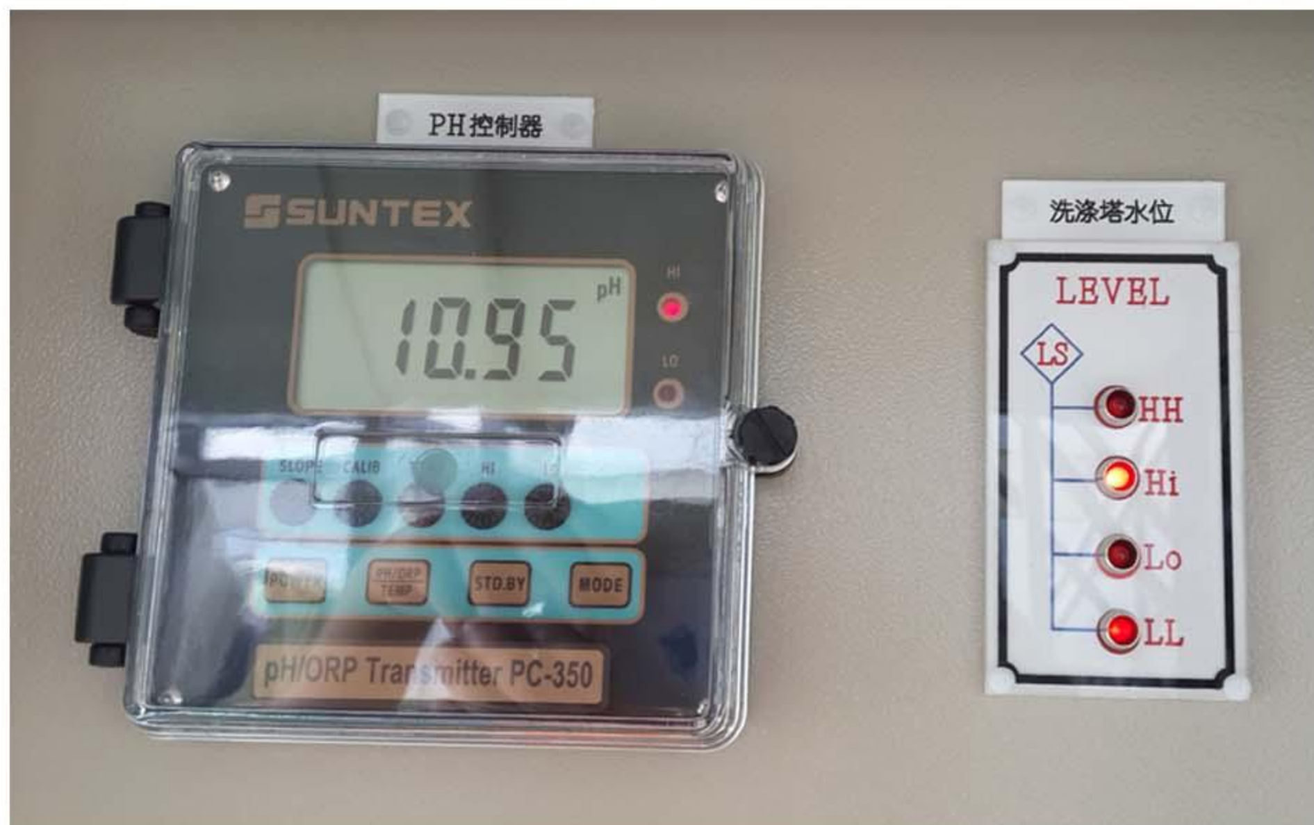
Control System of Scrubber Tower
