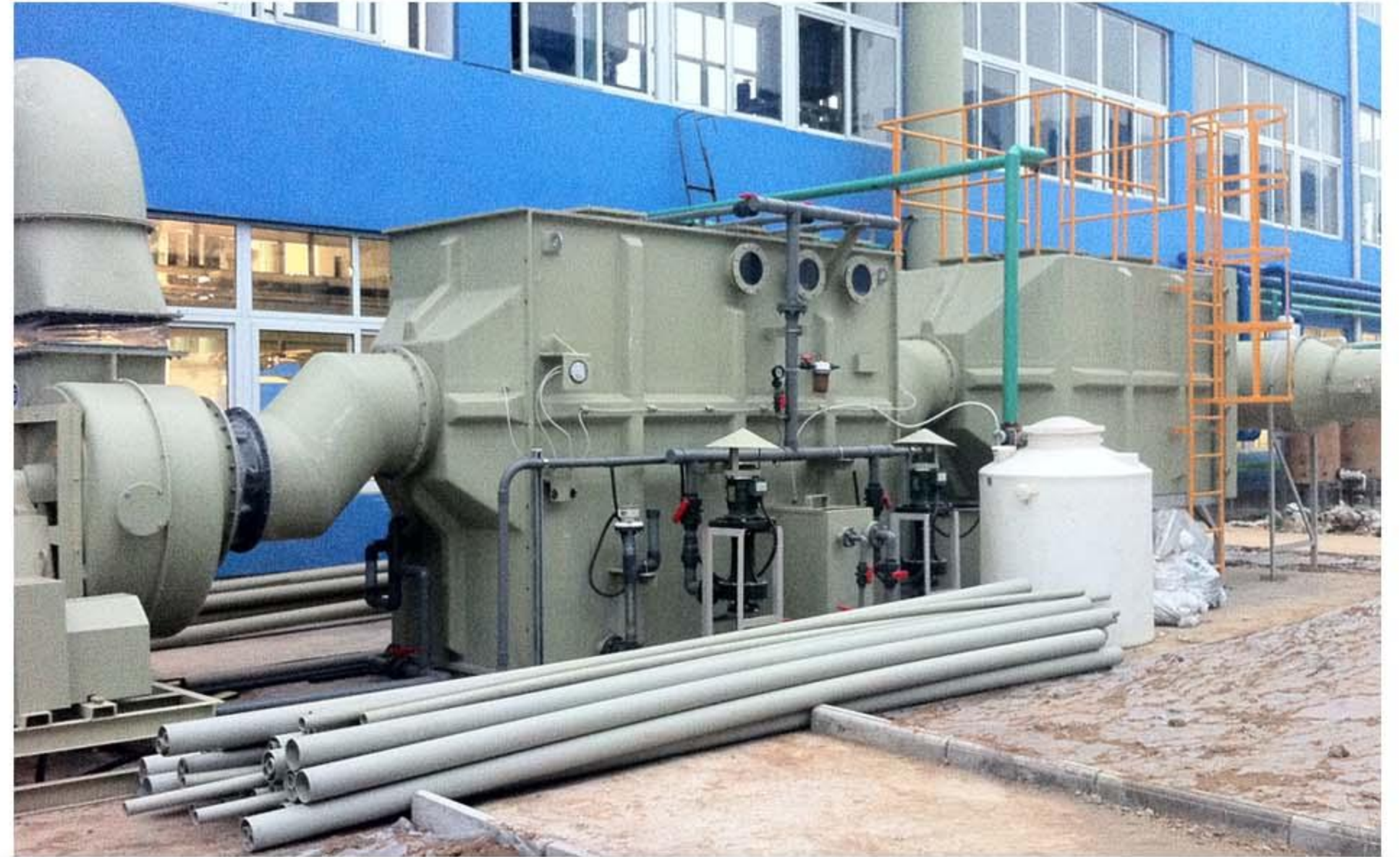
FRP Horizontal Scrubber Tower
