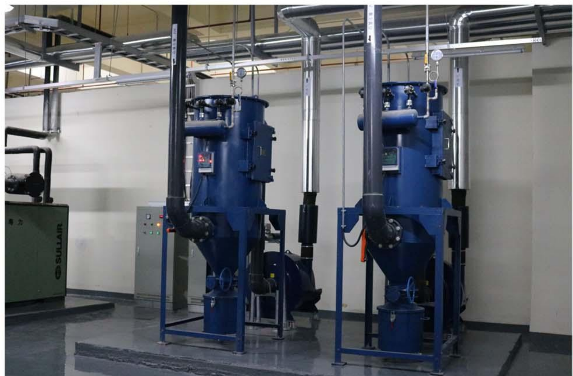
HV Vacuum Cleaning Dust Collection System for 8-Inch Wafer Plant - Zhengzhou
