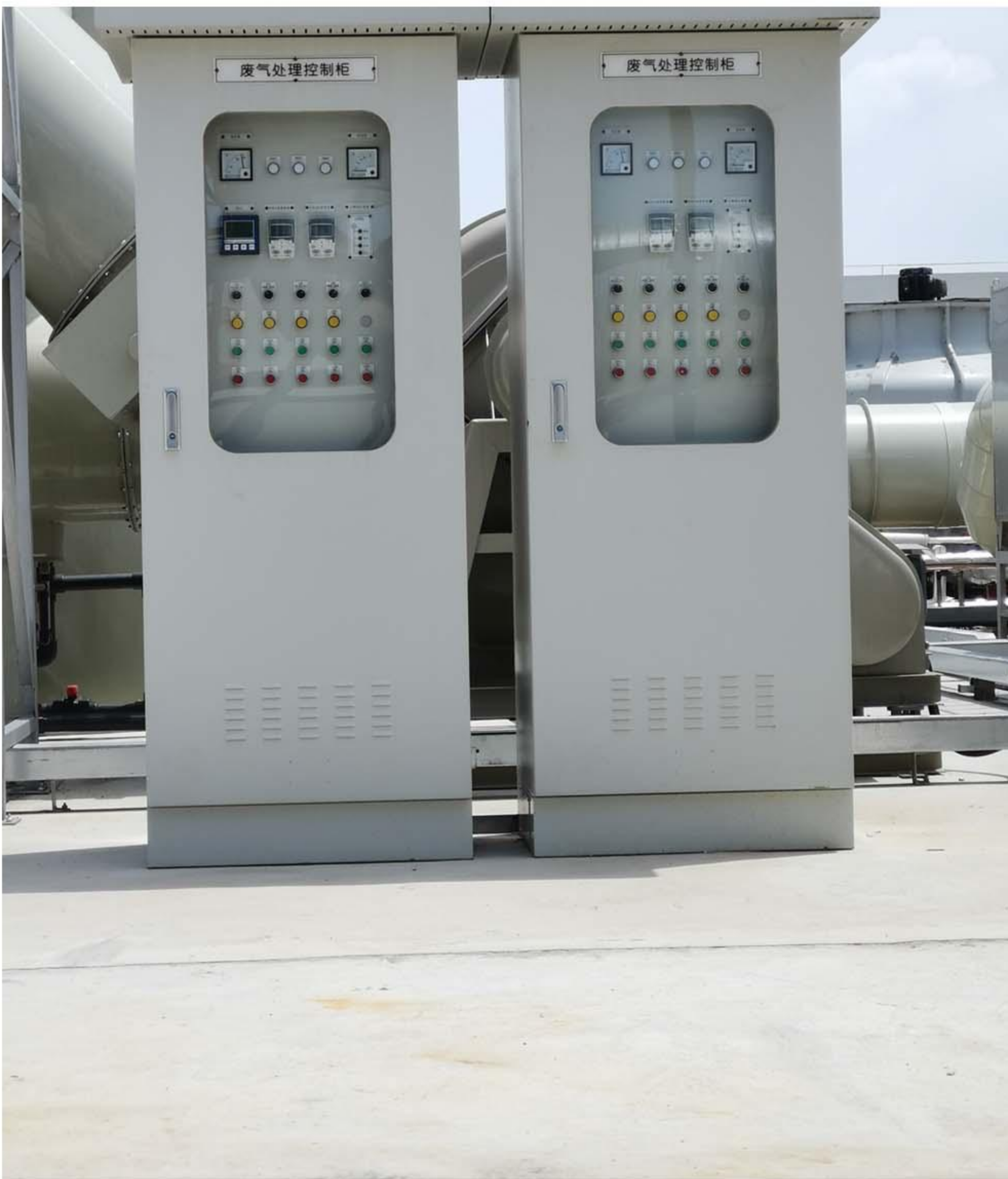
Outdoor Local Control Cabinet
