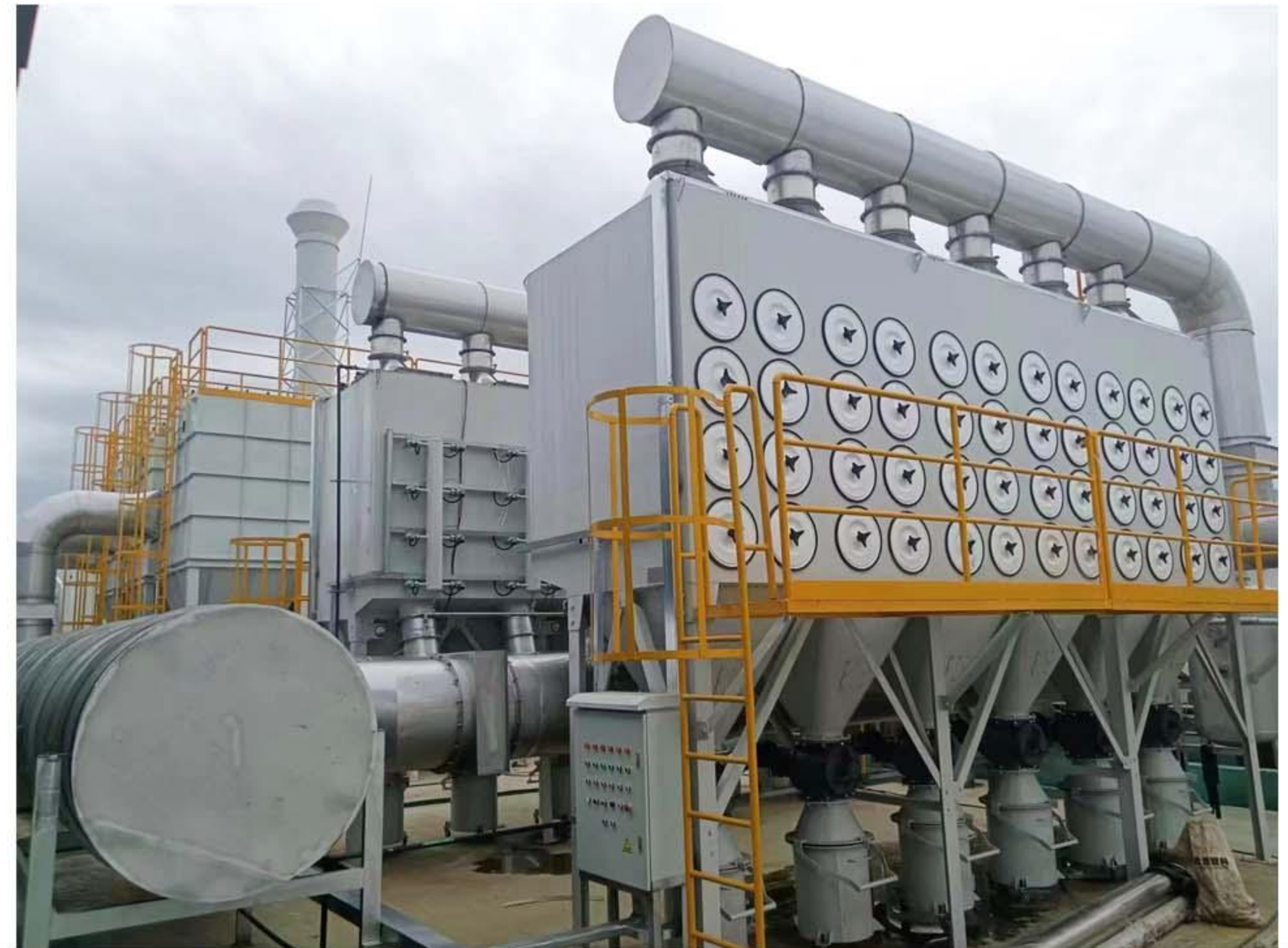
Photovoltaic Industry Dust Collection System - Chengdu
