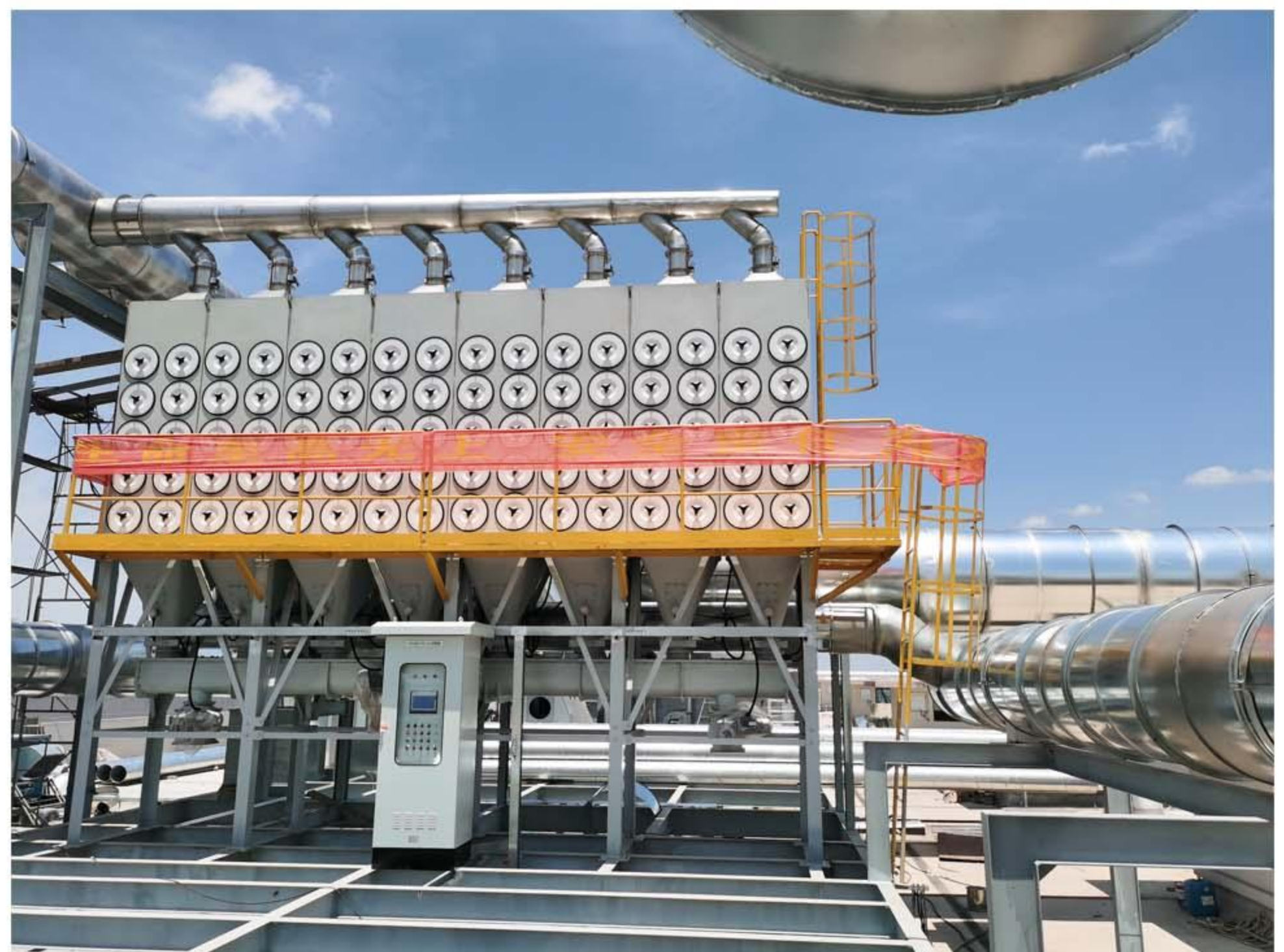
Resistor & Capacitor Industry Dust Collection System - Yiyang, Hunan
