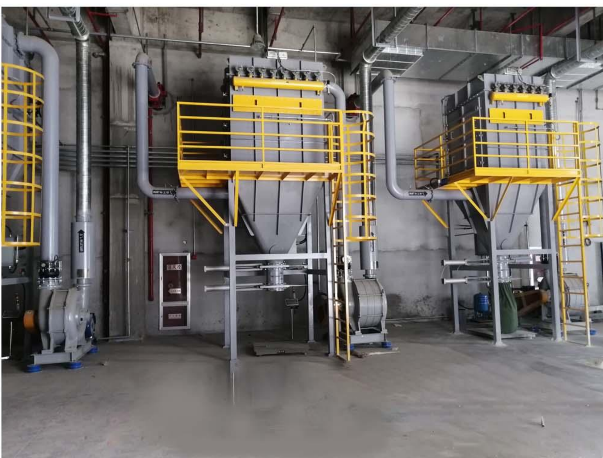
High-Pressure Dust Collection System for PCB Drilling Process - Changzhou
