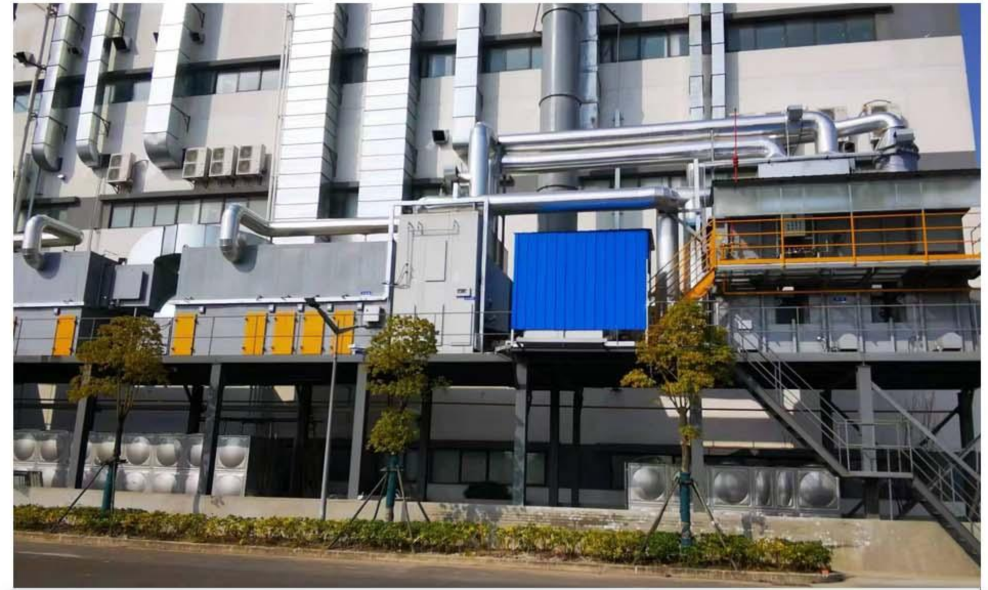
VOCs Treatment System with Zeolite Rotor + RTO for Laptop Shell Coating - Changzhou
