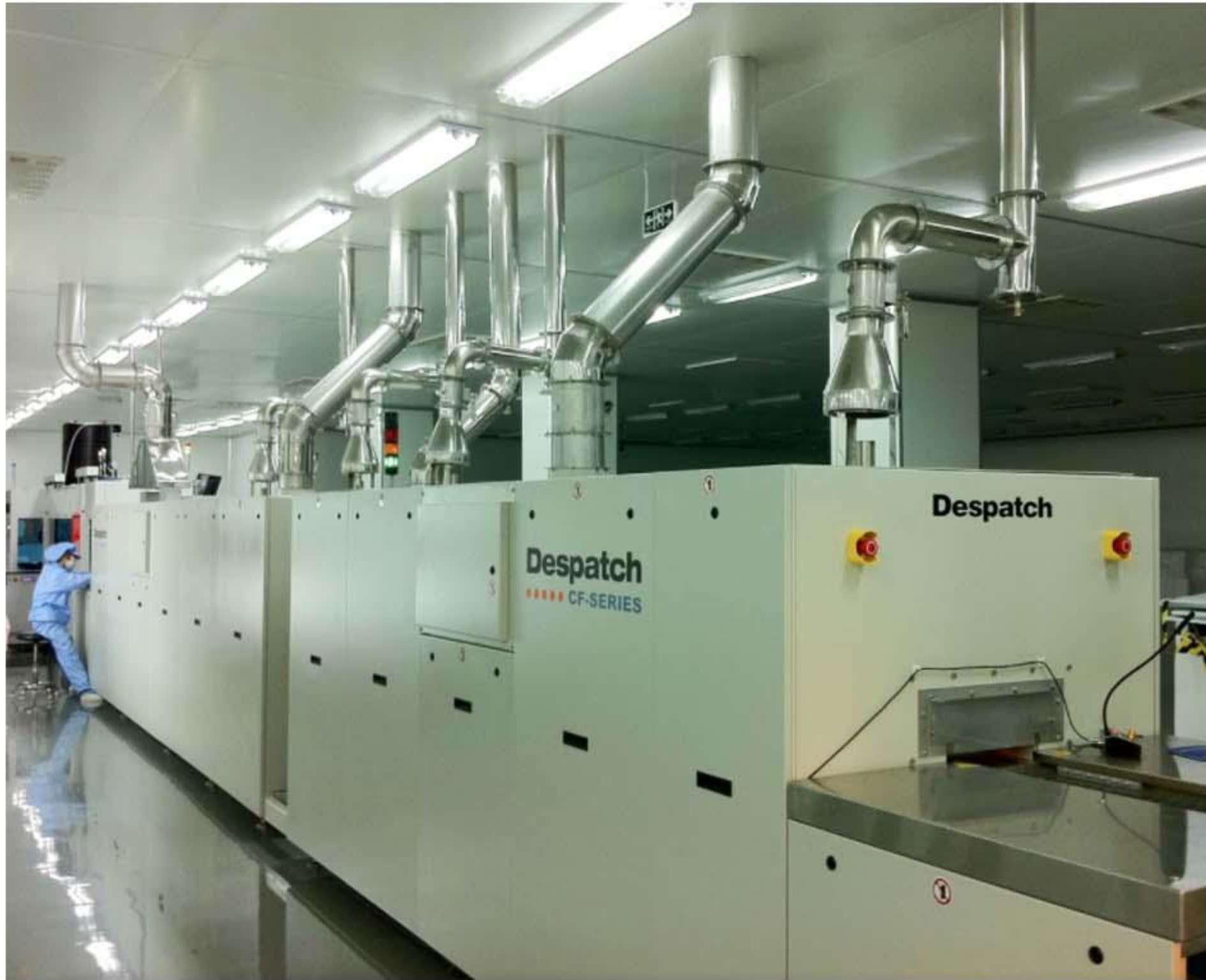
VOCs Exhaust Secondary Collection Piping Example Image (SUS304 Stainless Steel)
