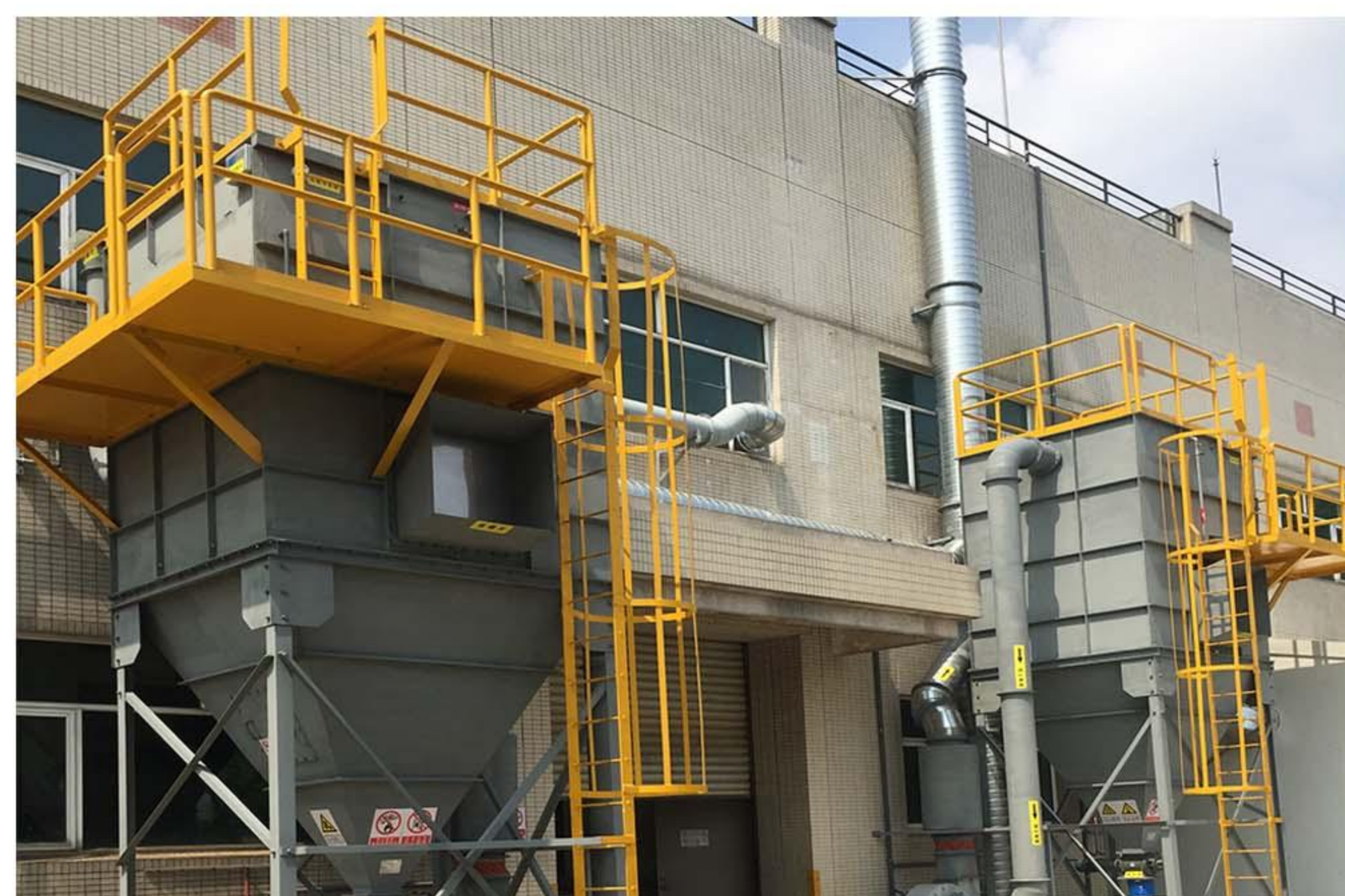
Explosion-Proof Dust Collection System for Chemical Industry - Suzhou
