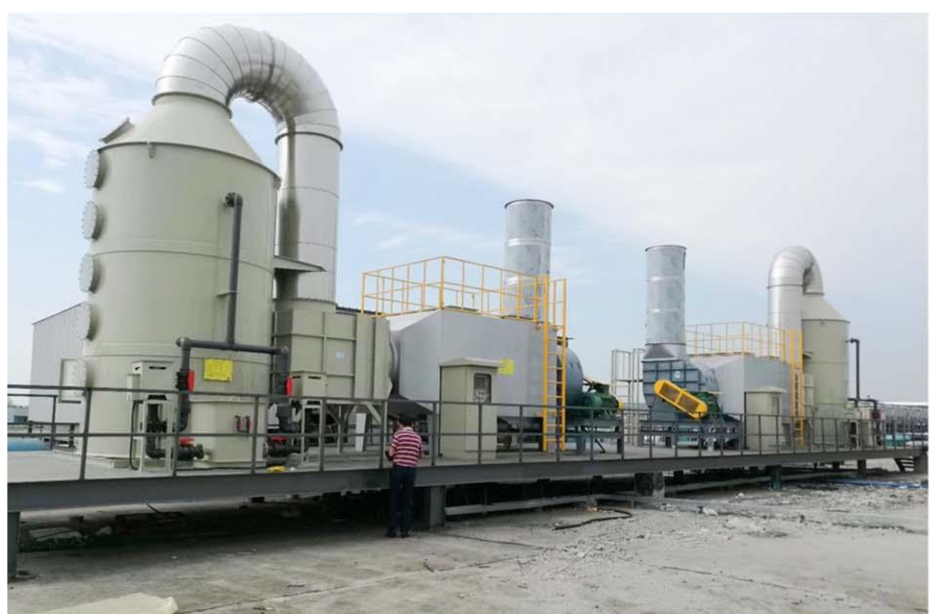
PCB Industry in Sichuan VOCs Purification System with Water Scrubbing + Activated Carbon Adsorption
