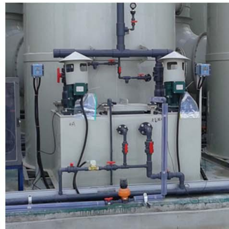
Spray Pipe Equipped with Water Pressure Gauge
