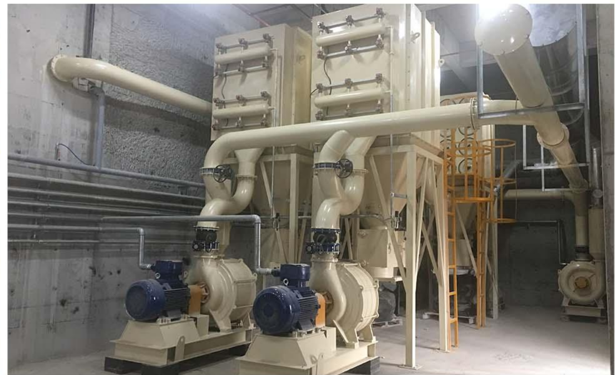
High-Pressure Dust Collection System for Drilling Workshop, PCB Industry - Huangshi, Hubei
