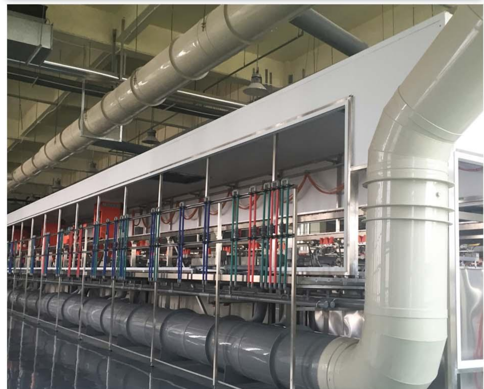
PTH Electroplating Line Acid & Alkaline Exhaust Collection Ducting Example Image (PP Plastic)
