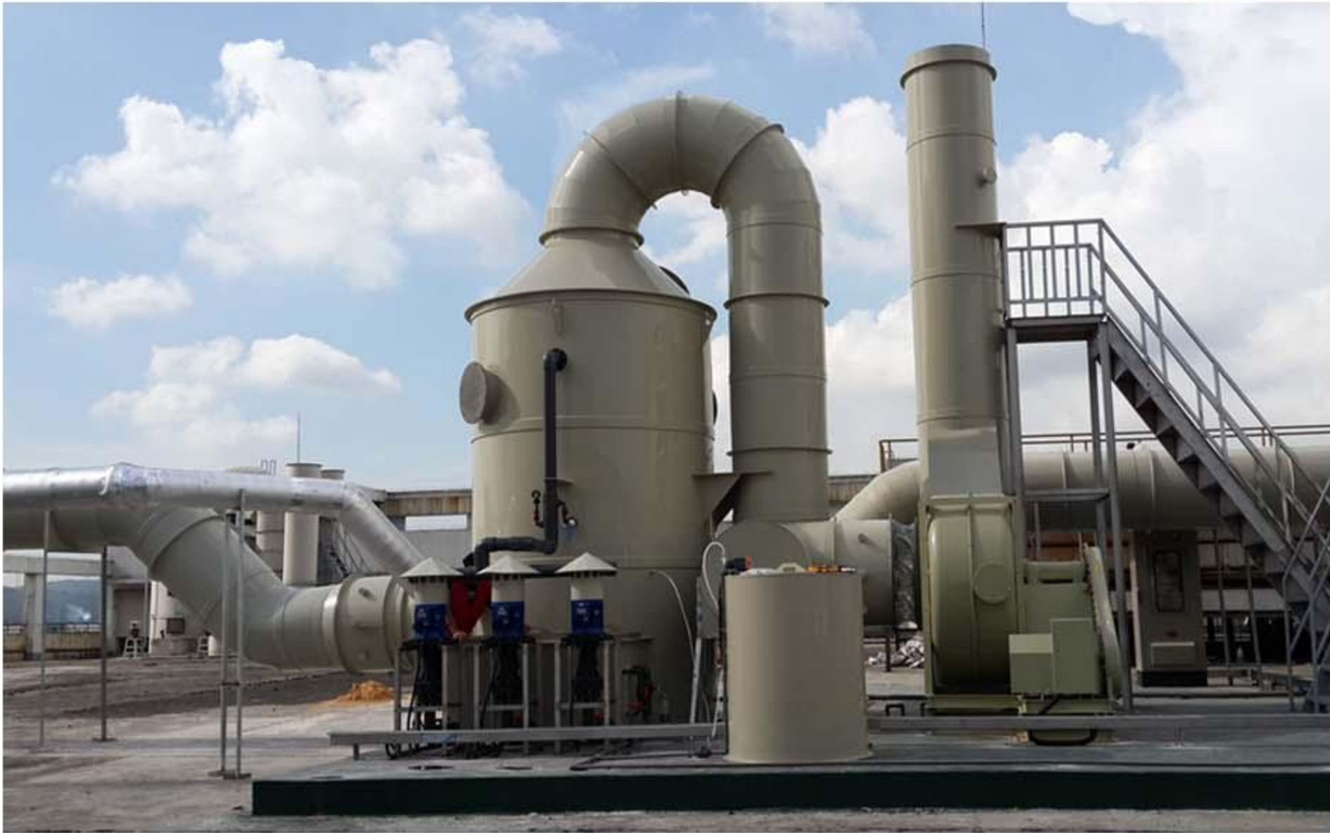
PP Vertical Scrubber Tower
