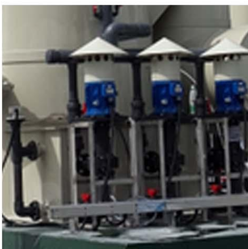
Dual-Pump Configuration (One in Use, One Standby)
