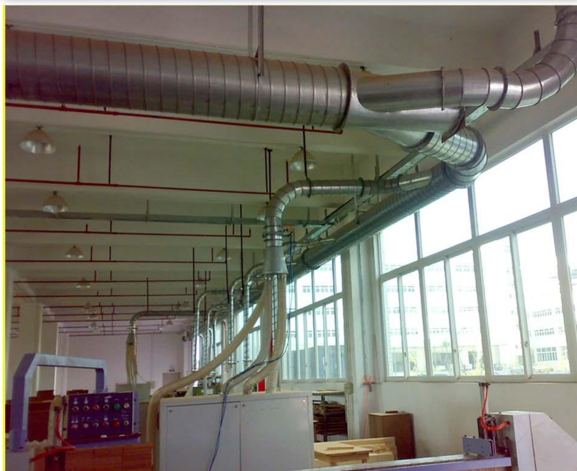
High-Speed Panel Cutting Machine Dust Collection Ducting Example Image (Threaded Galvanized Pipe)
