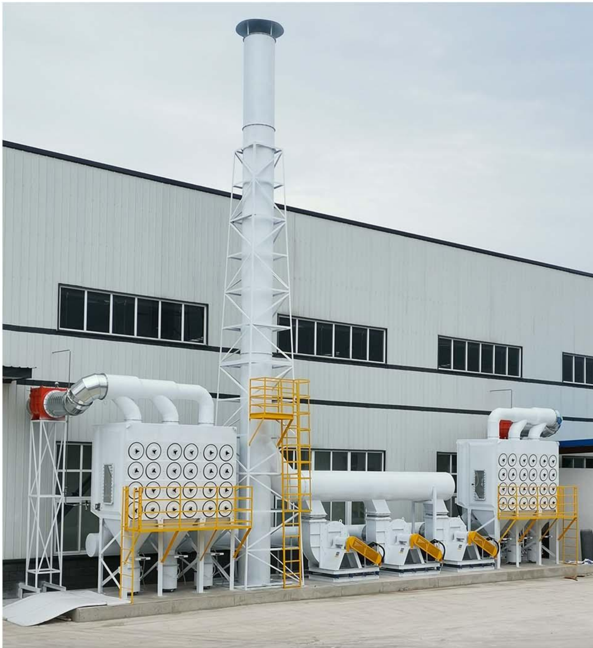
Semiconductor Thermal Spray Dust Collection System - Wuhu
