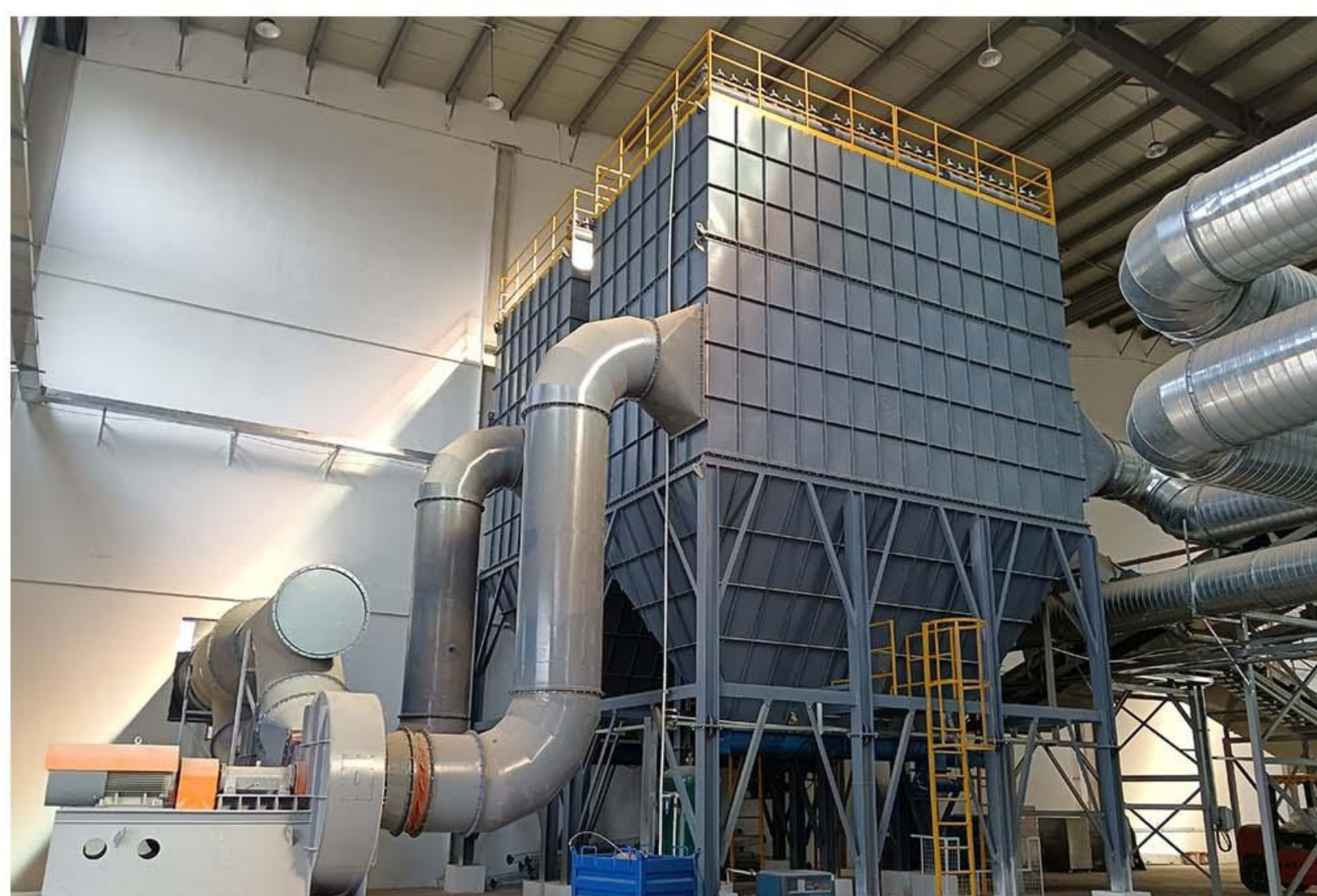
Urban Waste Sorting Dust Collection System - Yingtan, Jiangxi
