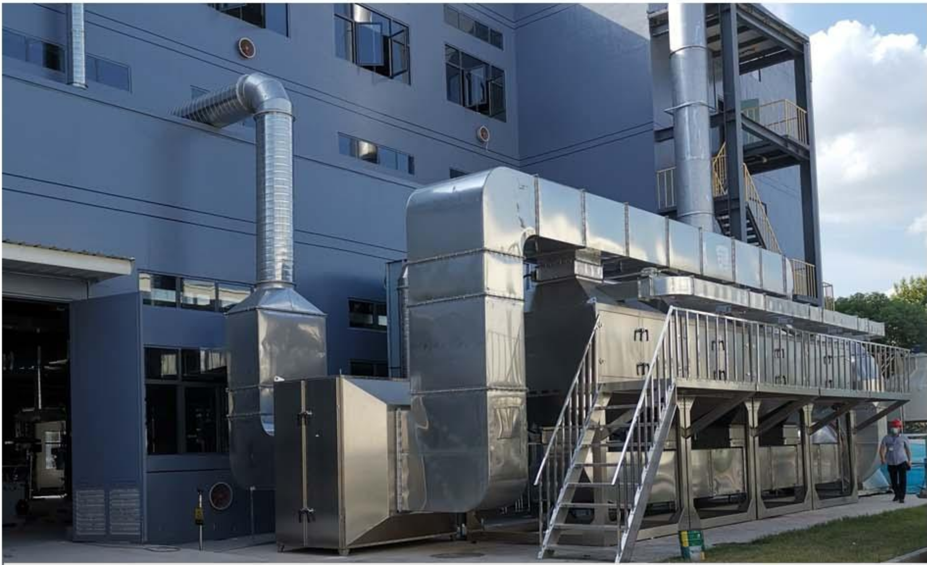
VOCs Adsorption - Desorption RCO Purification System for Coating & Chemical Industry - Wuhan
