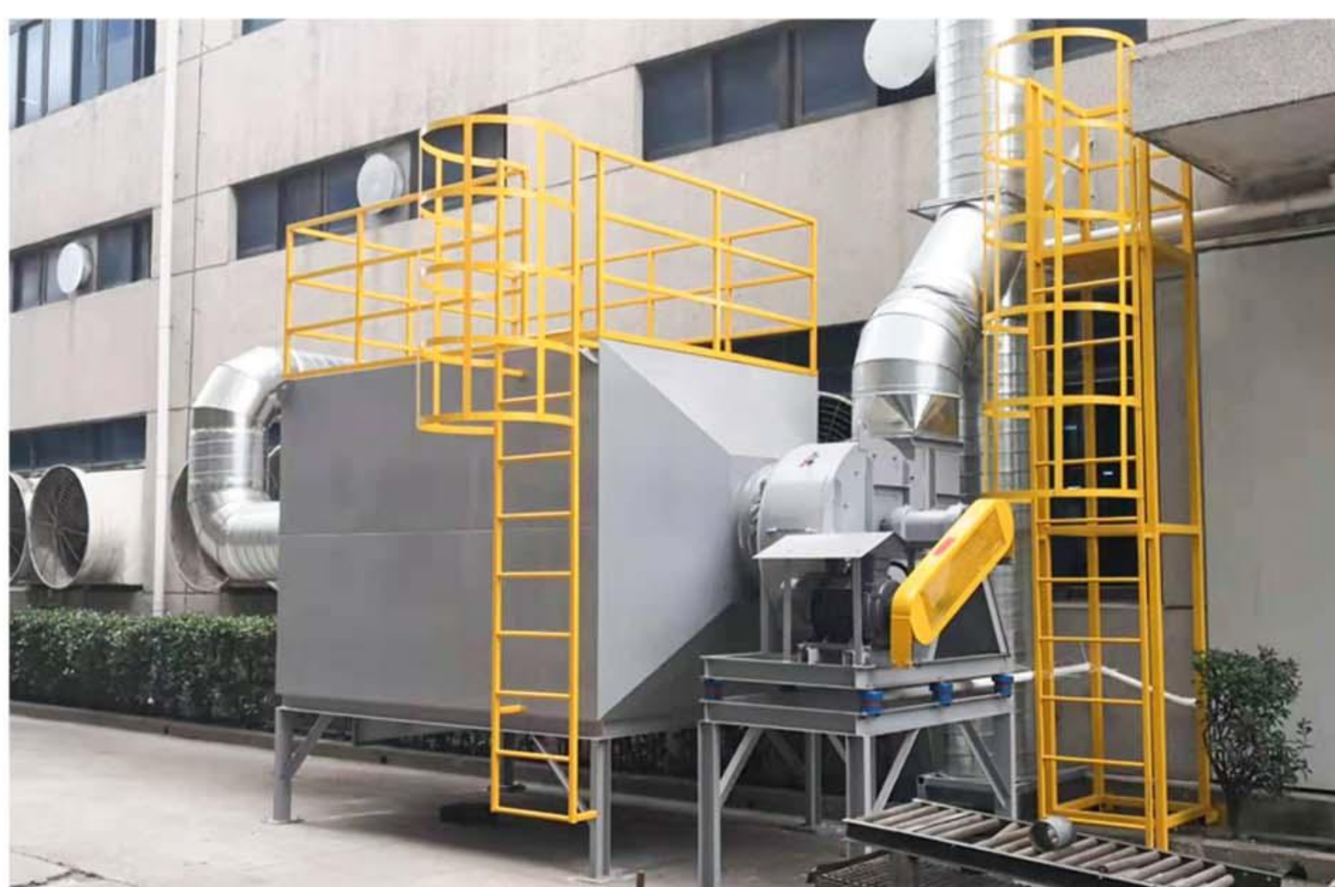
Coating Industry in Jiangxi VOCs Single-Stage Adsorption Purification System
