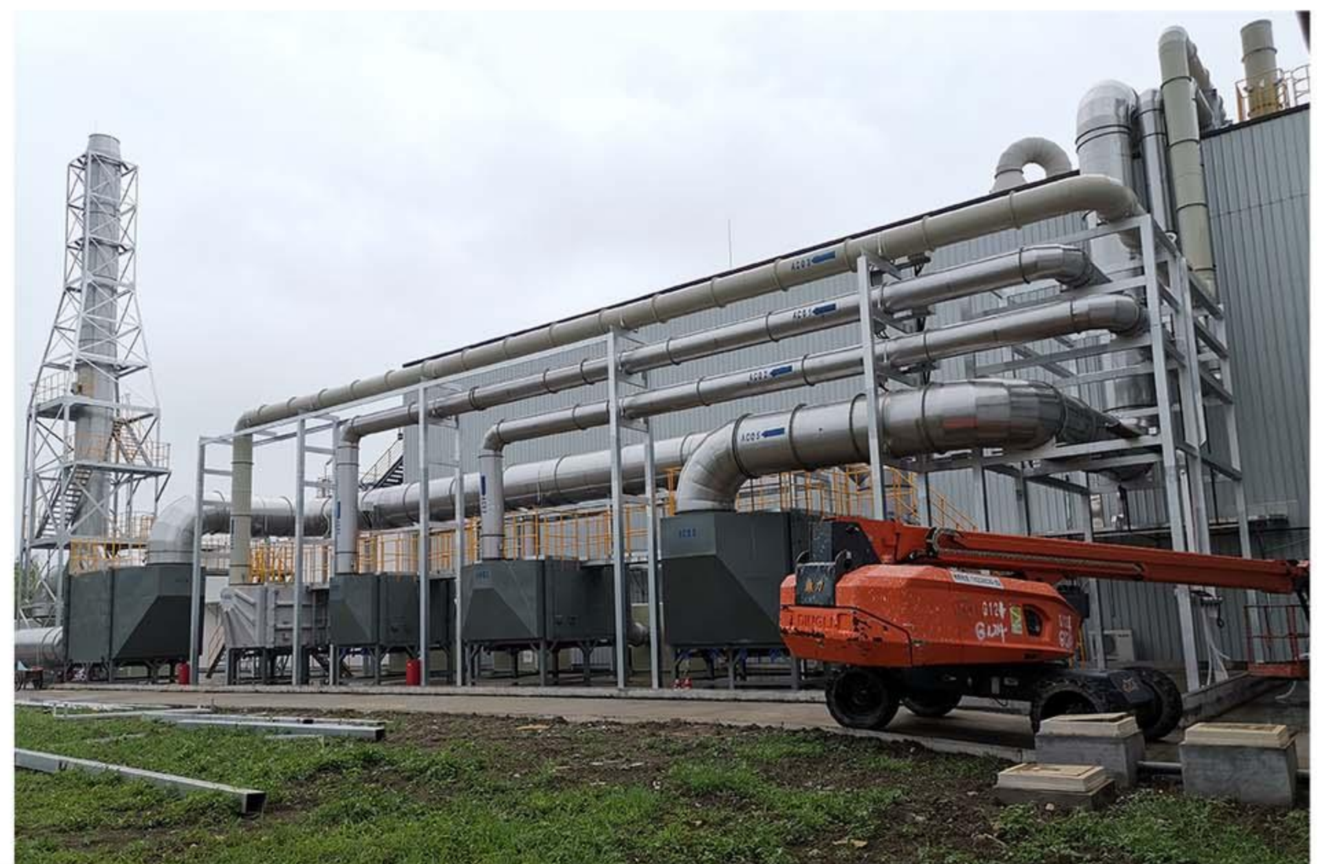
Chemical Industry in Suzhou VOCs Secondary Adsorption Purification System
